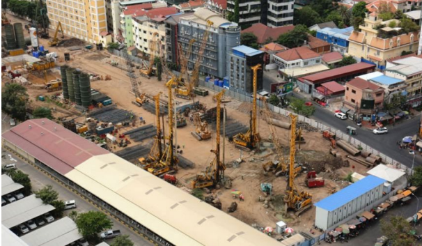
Aerial View of the Naga 3 construction site in Phnom Penh's Tonle Bassac commune.
