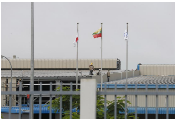
People working on the roof of a building in Thilawa Industrial Zone.
