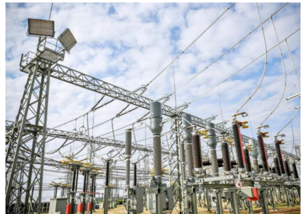
Three new substations were officially launched in Yangon Region on Saturday.
