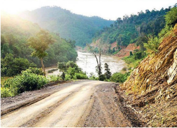
Part of the new road that will connect Dawei to the Thai border in Tanintharyi Region
