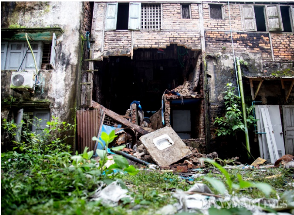
An old dangerous building in Yangon
